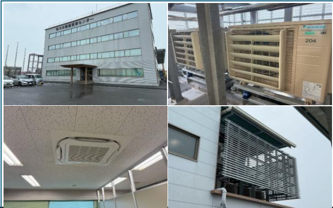
Energy Conservation in the Administration Building(Air-Conditioning System)
