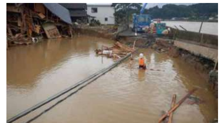
⑥ 堤防被災 (人吉市下薩摩瀬地先)
